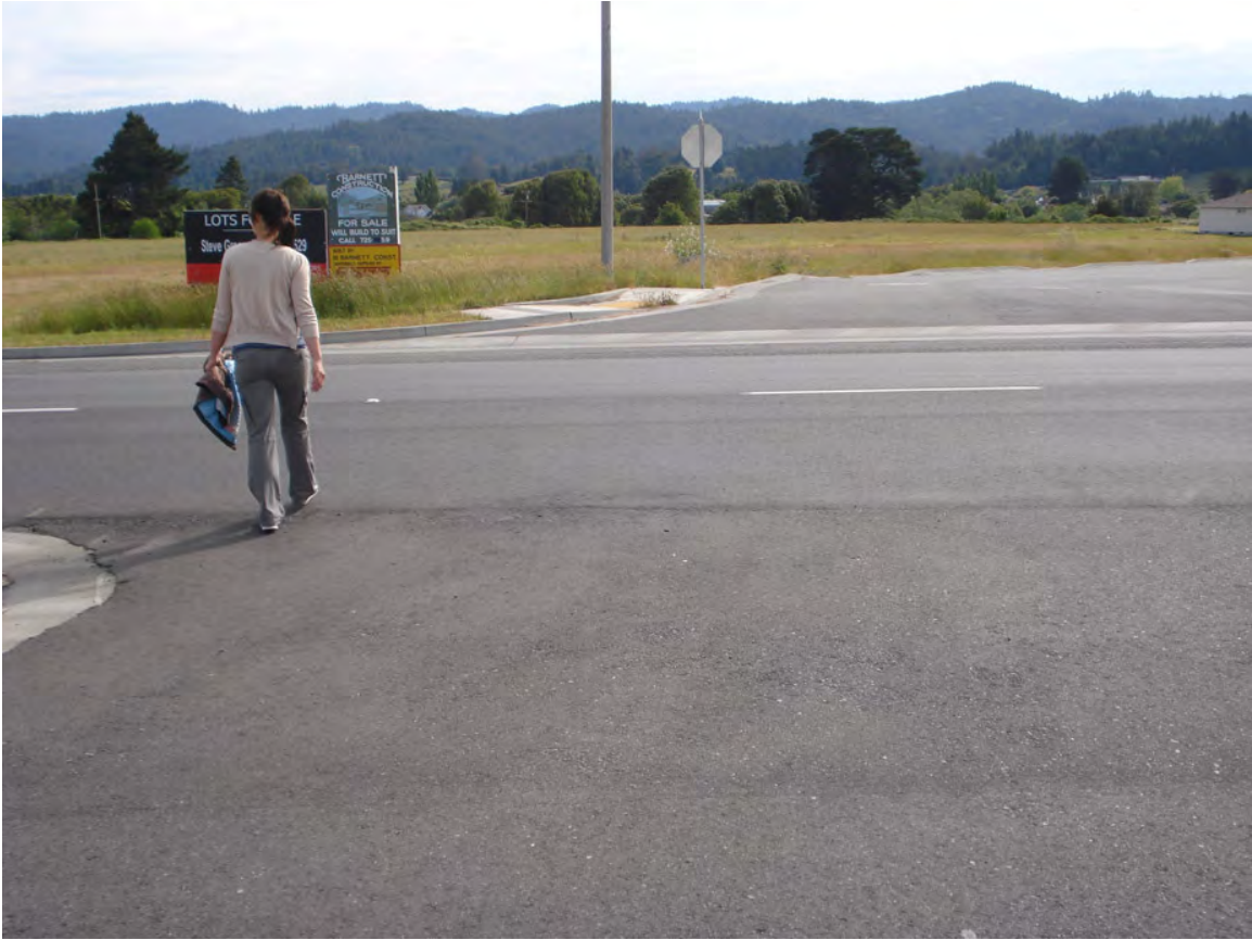
Ross Hill Road near Redwood Prep lacks crosswalks.
