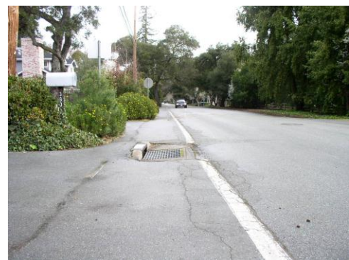
This drainage gate, located within a bike lane, forces cyclists to veer into the travel lane to avoid it.
